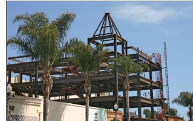
The building's distinctive tower was recently framed. When completed, the structure will house more than 20,000 square feet of office and retail.
