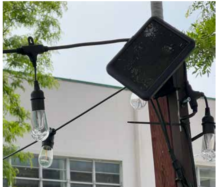
Self-contained low-voltage systems, such as solar or battery-powered lights, are encouraged for parklets
